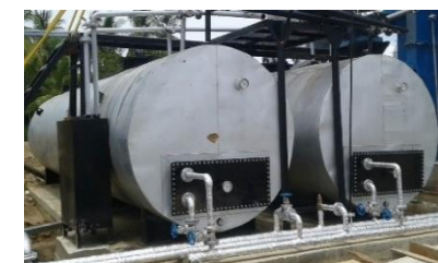
2 x Bitument Storage 25000 Ltr for AMP 1000
