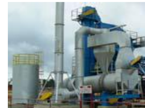
Fuel Tank, Exhasut Blower, Dust Collector and Dryer
