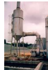
Wet Cyclon Dust Collector
