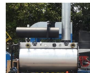
Hot Oil Heater
